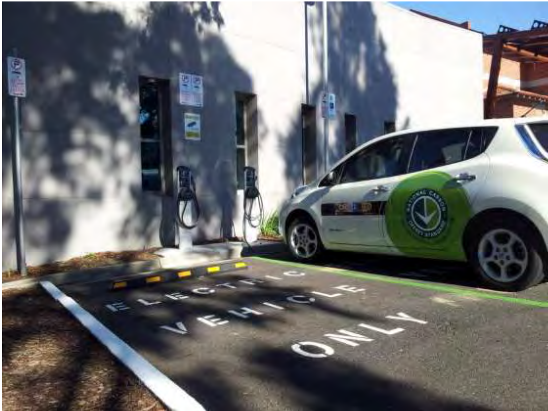
Figure 1 Recharge Station, Moreland City Council offices
